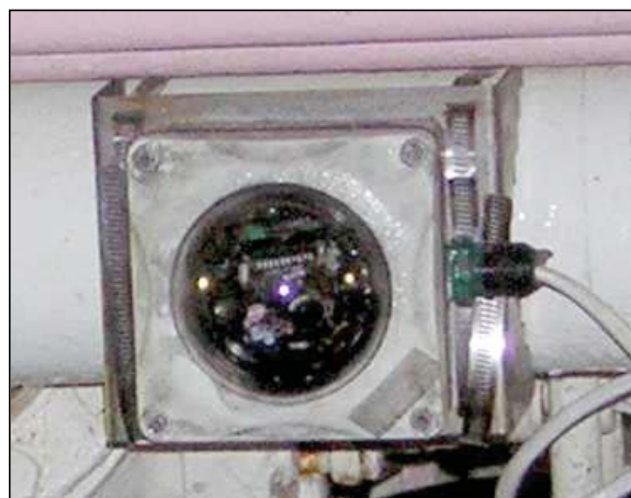
Figure 3. Photograph of an installed CCTV camera on F/T Seafisher encased in a cast aluminum armoured dome, showing stainless steel mount and band straps.
